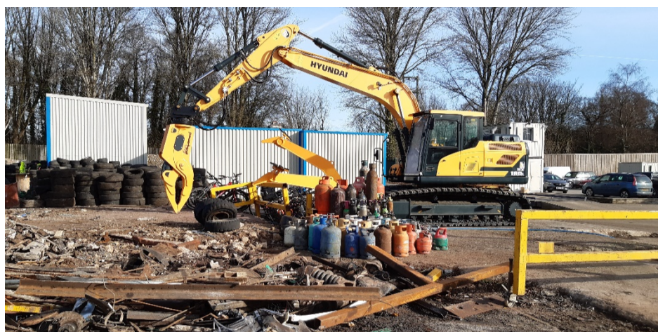
Image 3 - showing removed and quarantined gas cannisters from stockpiles
