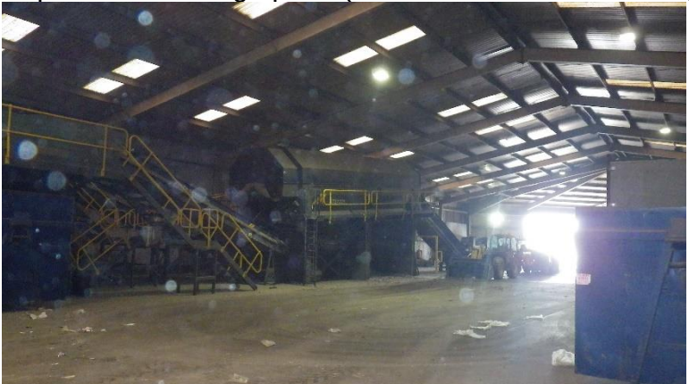
Trommel and associated treatment kit including magnet, blower, eddy current separator etc.
