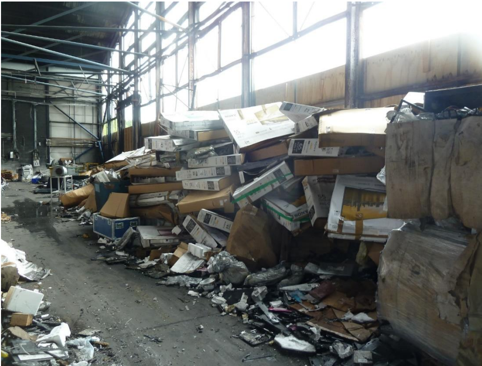
Photograph showing some of the waste stored in the damaged building. Waste is not authorised to be stored in this area as the building has not been maintained to prevent the ingress of water. (Photo ref:P1030373)
