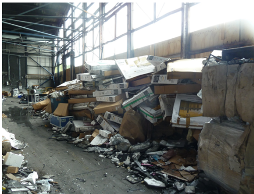
Photograph showing some of the waste stored in the damaged building. Waste is not authorised to be stored in this area as the building has not been maintained to prevent the ingress of water. (Photo ref:P1030373)
