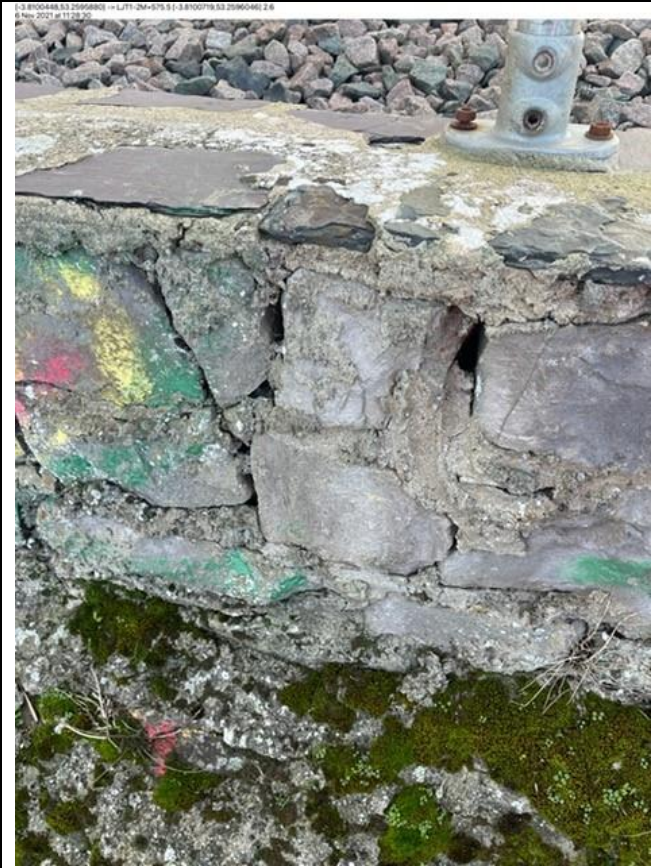
Capping repairs required
