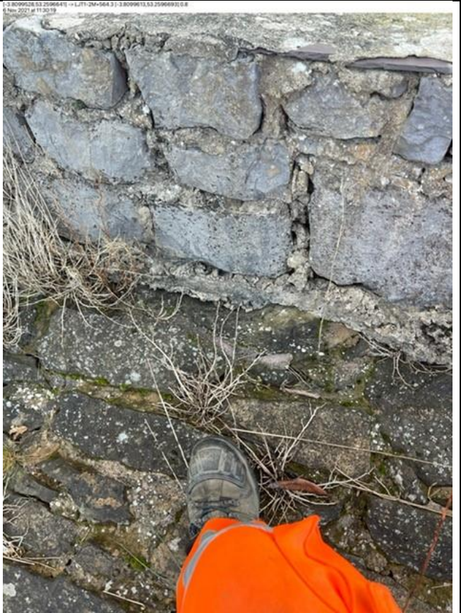
Capping repairs required
