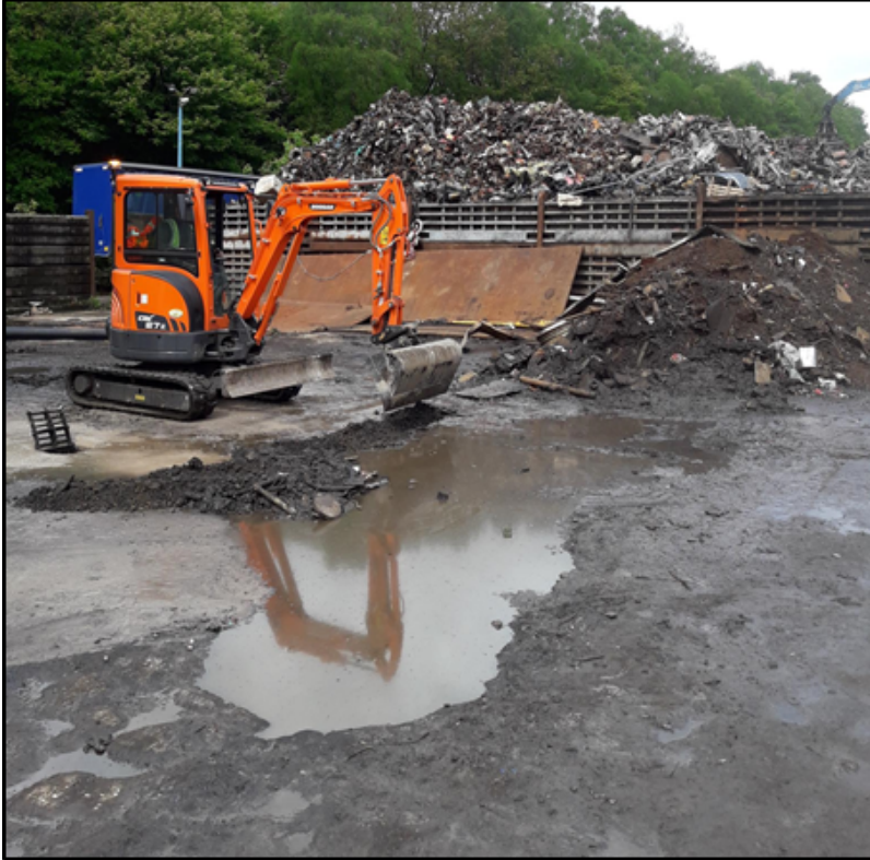
Picture 4 – showing an area of weakened infrastructure in the yard, taken on 08/05/18
