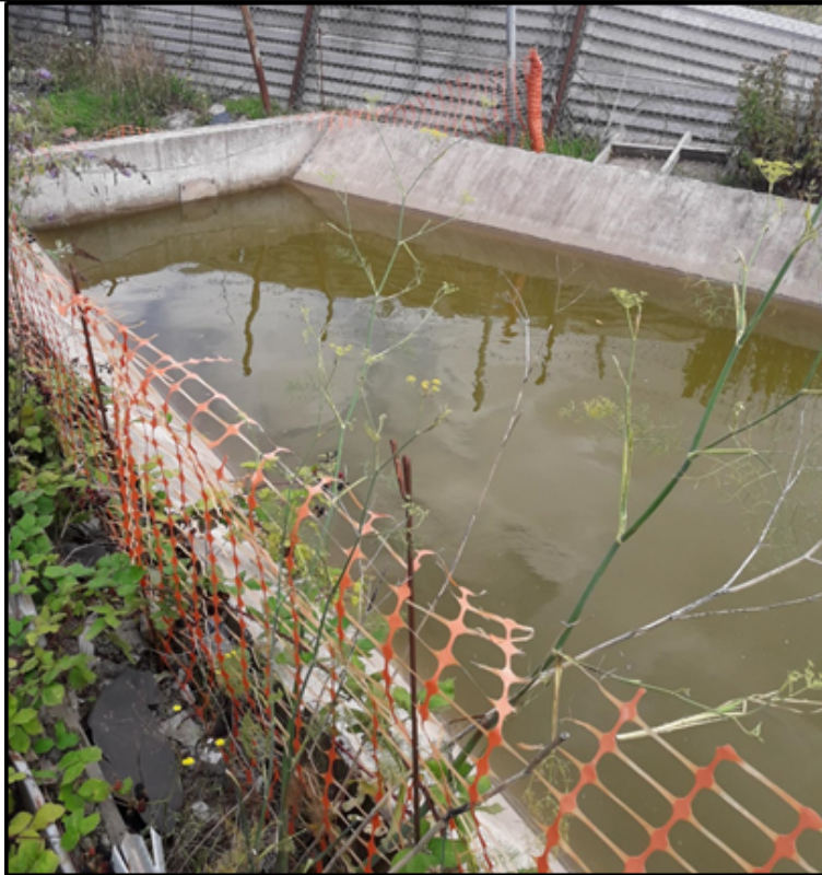
Picture 1 - showing surface water pool at the rear of the yard
