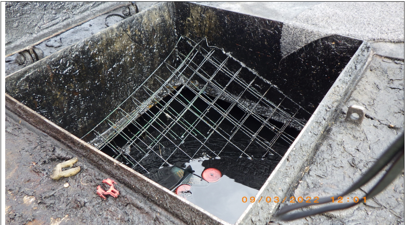
Photograph showing a tank containing oil which is almost full
