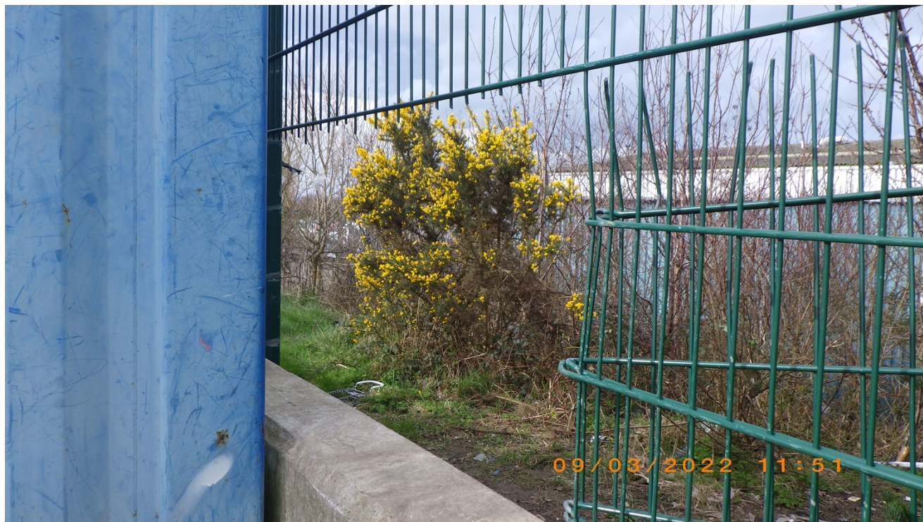
Photograph showing broken fence on permit boundary
