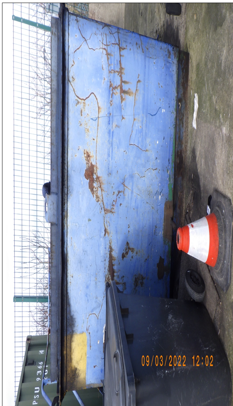
Photograph showing waste oil tank
