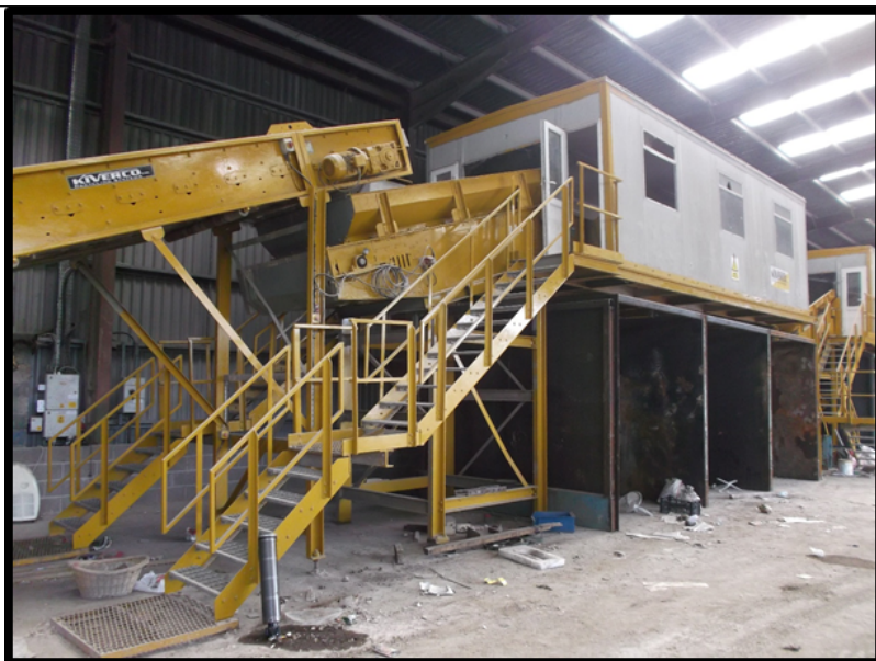
Picture 2 – showing new machinery inside building
