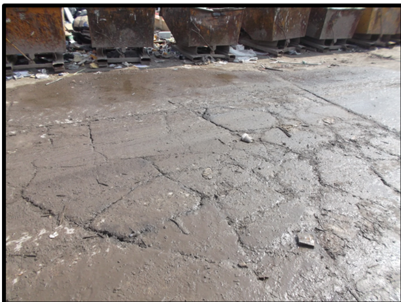
Picture 3 – Showing cracks in the concrete
